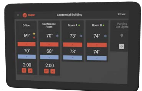
BAS Trane Tracer® Concierge® Controller with mobile access (wired or wireless Air-Fi®)
