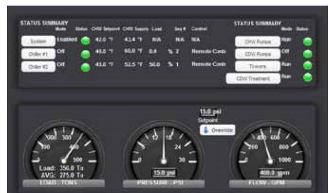
Tracer dashboards use an easy-to-interpret graphical display to report current operating conditions and energy usage.
