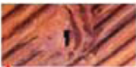
INTERNAL PITTING Caused by an abnormal presence of aggressive elements in water.
