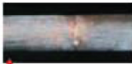
TUBE SUPPORT WEAR Caused by the tube/support contact. Although this phenomenon is quite rare, it must be quickly detected.
