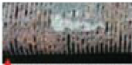
EXTERNAL CORROSION Caused by air intrusion.
